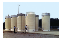
Dry Storage Casks
